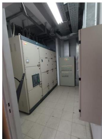
FIGURE 2. Low Volt Main Distribution Panel (LVMDP)
